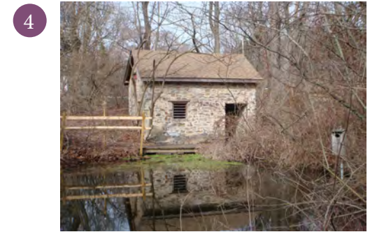
4 Spring House - The historic spring house is in decent shape. Could be restored and used as an education tool.
