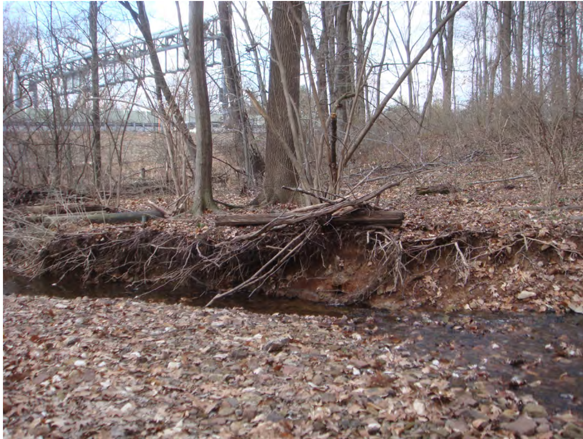
Figure 50: Image showing the deep incision into the creek bed and the heavy streambank damage caused by years of uncontrolled stormwater flows.
