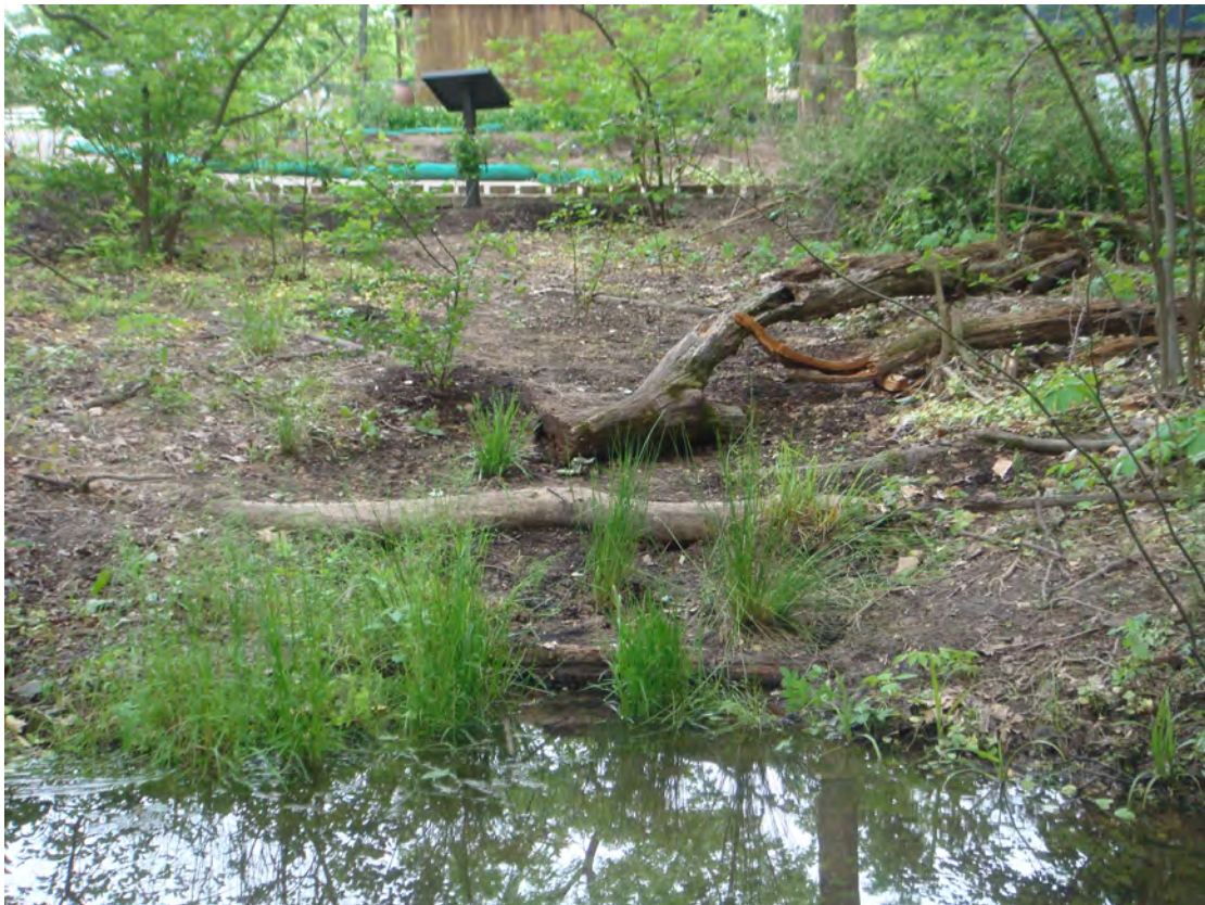
After - Closeup view of stabilized erosion channel after planting. Existing logs from the site used to create the sills and other logs replaced back on top in order to keep the natural habitat and look intact.
