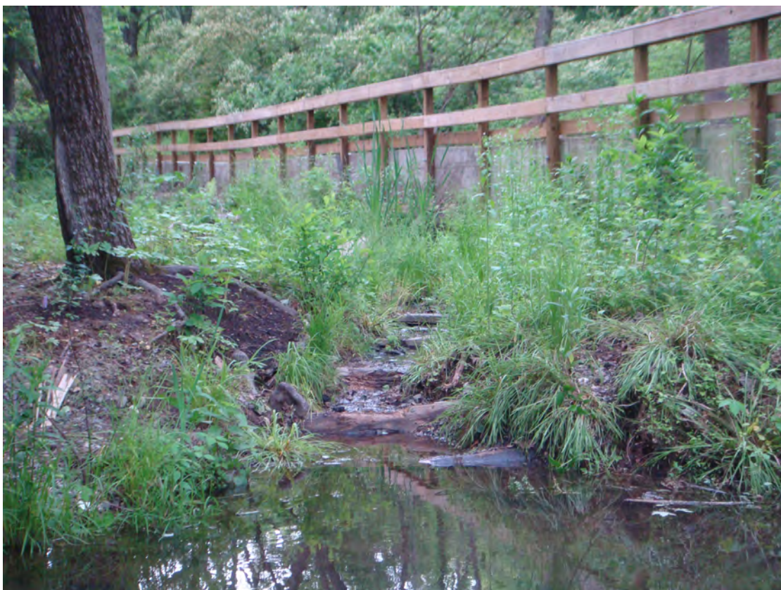
After - Rock and log sills added to stabilize and fill in eroded channel. Soil added to cover exposed roots and native plants added to help stabilize the soil and provide habitat. Tadpoles have already taken up residence in the newly created pools behind the sills.
