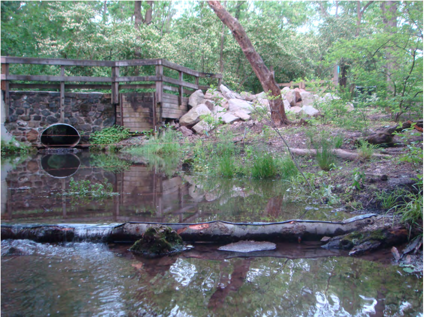
After - View upstream showing the installation of a sill log across the stream. The stream is heavily incised, so sill logs are being used to help bring the stream bed and water level back up to historic conditions, which will help return the system to its natural floodplain.
