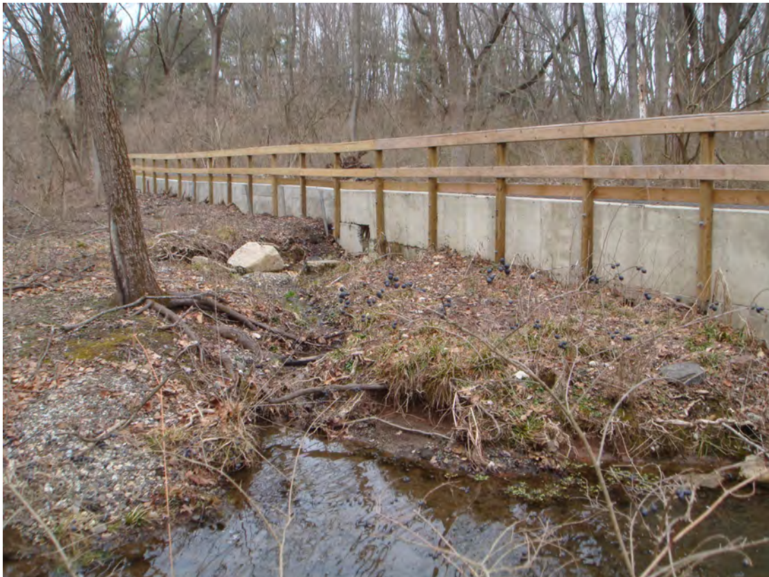
Before - Eroded stormwater channel leading to creek. Roots of black walnut exposed.
