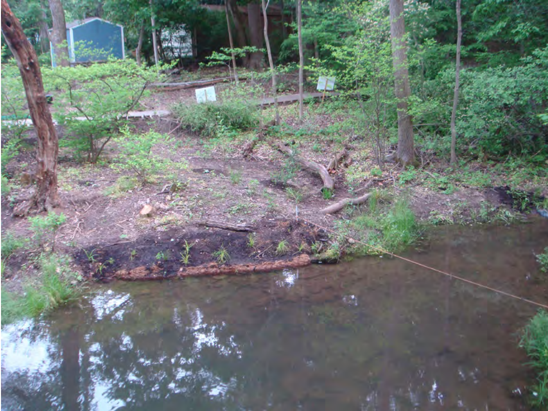
After - Exotic plants removed and rain garden system installed above path. Eroded channels stabilized with sill logs, filled with soil and planted with native plants. Streambank stabilized with coir log and coir fabric and planted with native grasses, sedges and rushes.
